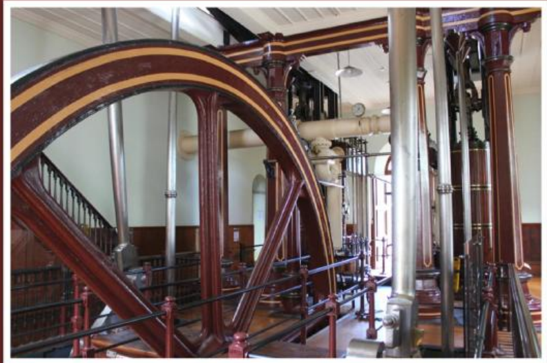
The 1877 beam engine at the former Auckland Waterworks and Pumping Station at MOTAT, Western Springs.
