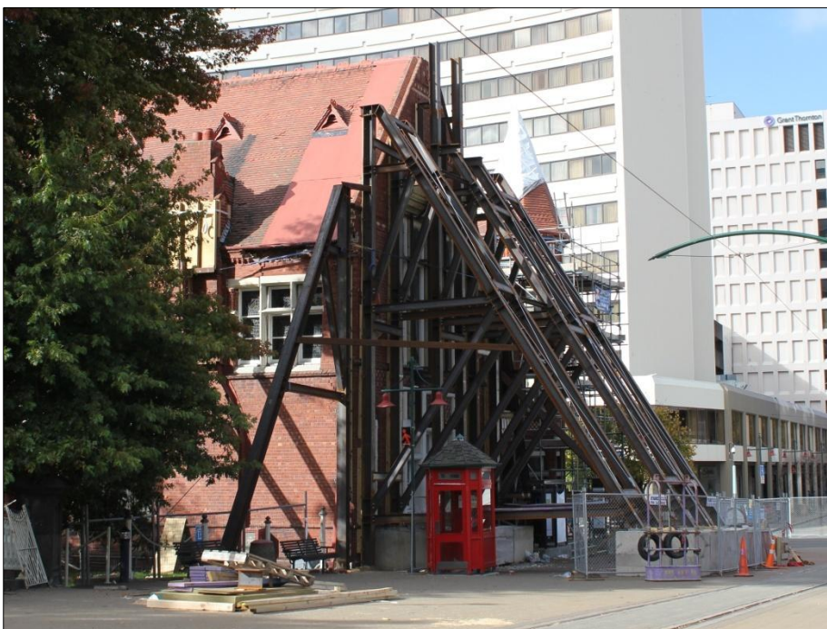
Possibly the most propped building in Christchurch Samuel Hurst Seager's 1887 former Municipal Chambers : Our City O-Tautahi awaits attention.
