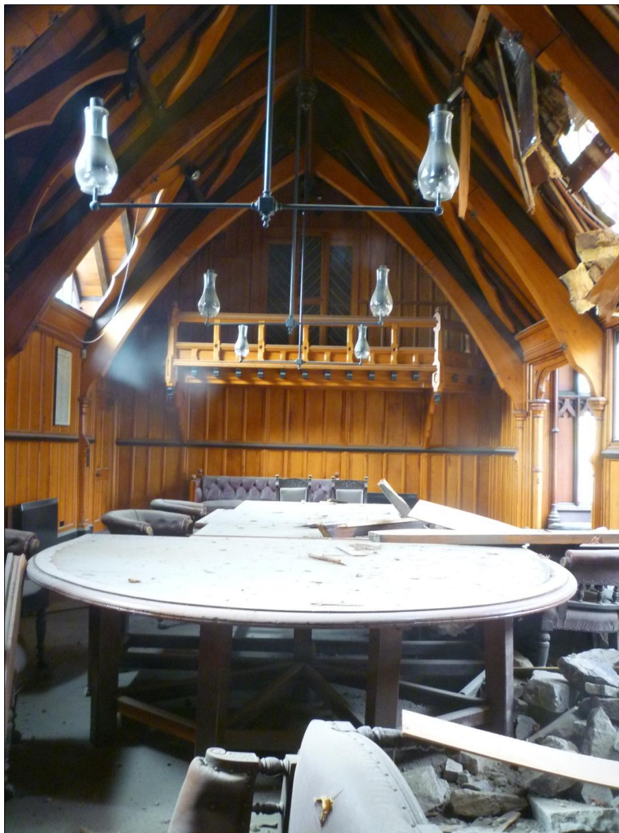
Damage to the Timber Chamber, the first part of the Canterbury Provincial Buildings, completed in 1859.
