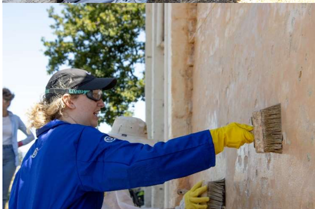
Alex (top) and Laura limewashing a wall during the Longford Academy Course in February 2023
