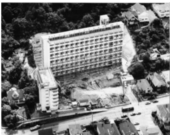
The flats under construction, 1958 . Ref: EP/1955/2193-F and EP-Industry-Housing-State-02. Alexander Turnbull Library, Wellington
